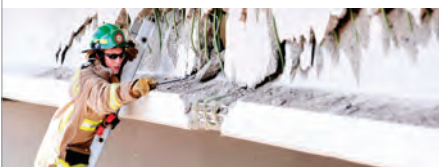
Mechanical - Impact Damage
