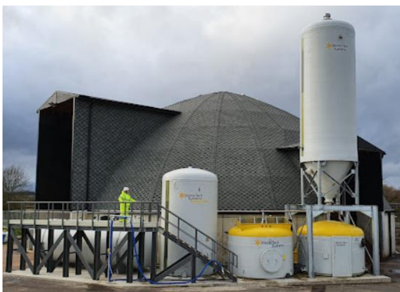
50m 3 silo installation in Newport Pagnell, England
