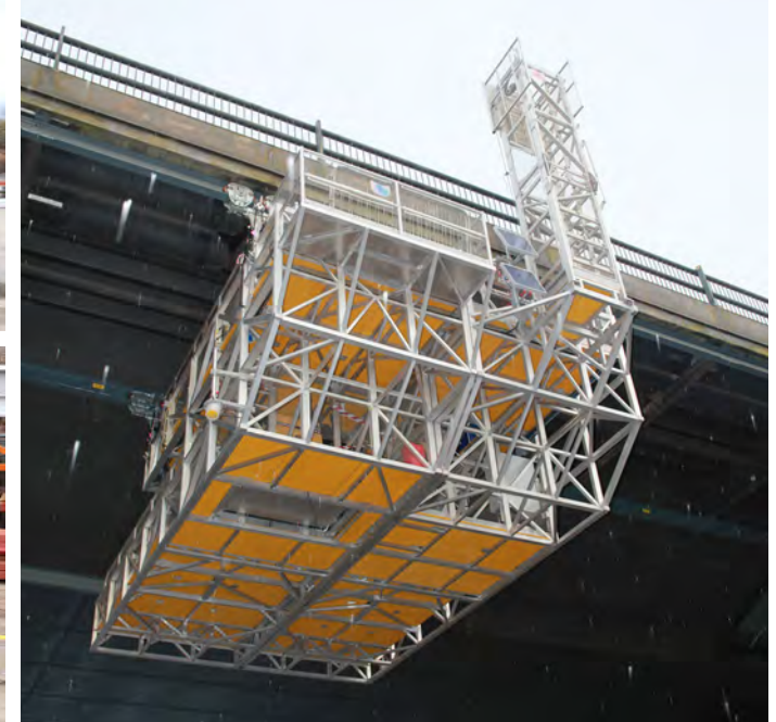
Erskine Bridge Underdeck Gantry
