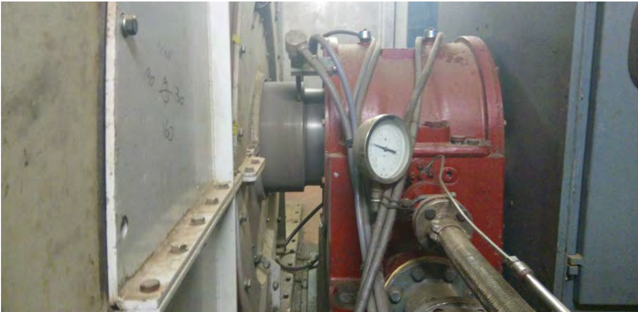
Figure 3. The shaft between turbine and generator.
