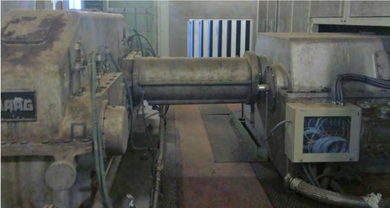
Figure 2. The main turbine.
