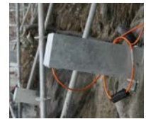
Rock anchor monitoring
