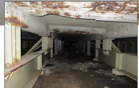
Spalling transverse beams to soffit under deck joints
