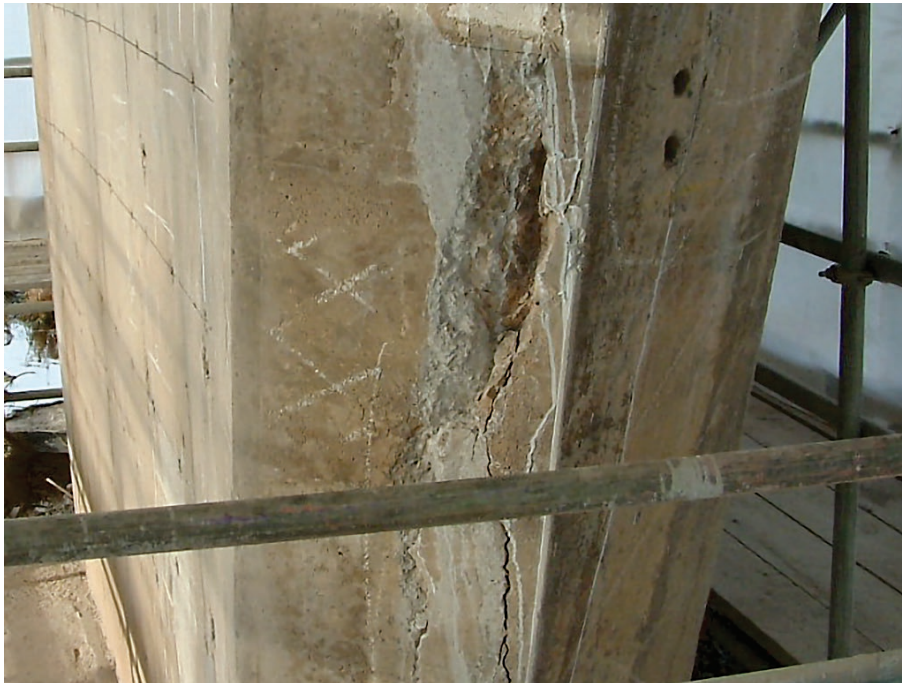
LEFT: Figure 2 – cracking of bridge pier prior to repair in 2007.
