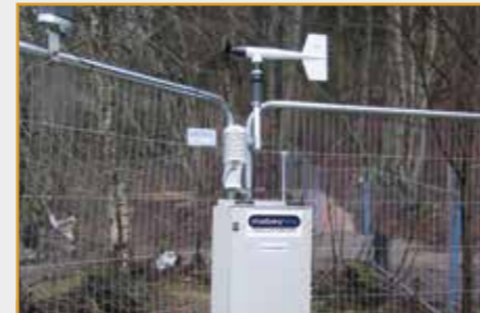
Enviroguard units are fully installed and commissioned by our expert engineers.
