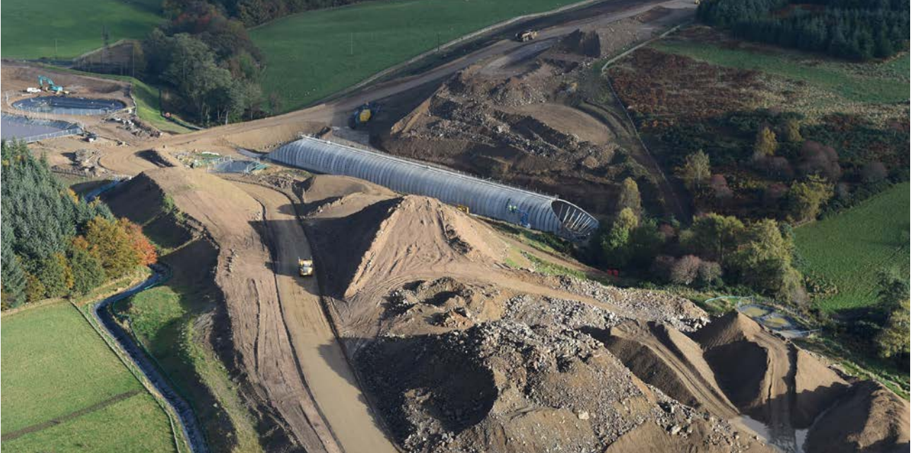
Aberdeen Western Peripheral Route PS02 and PS41A (asset BEBO® Arch C42T/9 - Span 12.802m - Rise 8.026m)
