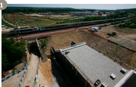
1 - Prefabricating the structure next to the track and positioning the driving nose
