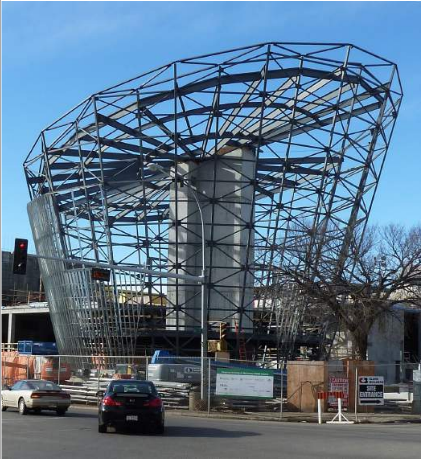
Nearly 1,000 CAST CONNEX Universal Pin Connectors were used in the space frame of the Physical Activity & Wellness Centre at The University of Alberta.
