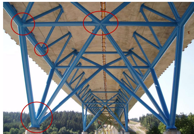
Figure 6: The Sankt Kilian Viaduct, completed in 2006, utilizes cast steel nodes at the locations identified to address multiplanar tubular connections.
