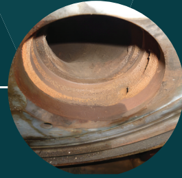
Eroded water-cooled valve seat pockets
